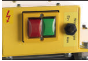
Switchable water pump for wet cutting.
